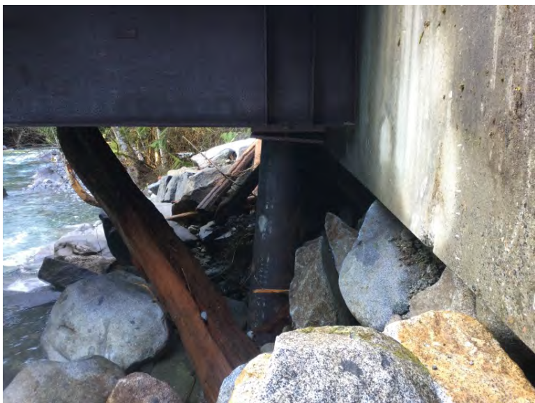
Upstream woods abutment pipe column leans to fill side
