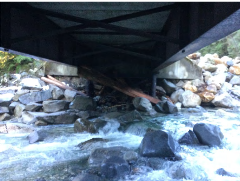
Upstream woods abutment has settled
