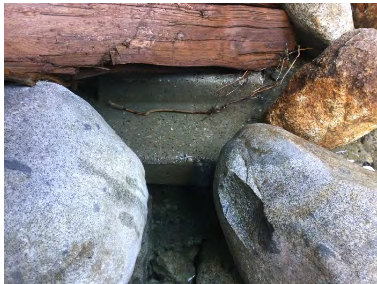
Upstream woods footing scour
